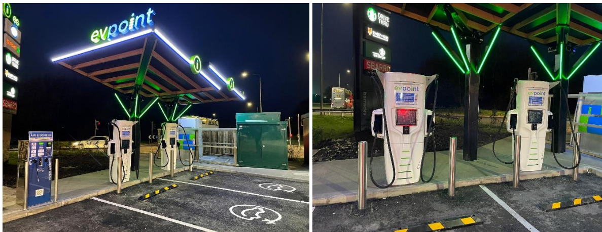
Photo of New 175Kw Ultra Rapid Chargers Installed at Euro Garage Petrol Station Barracks Road Burnley.
